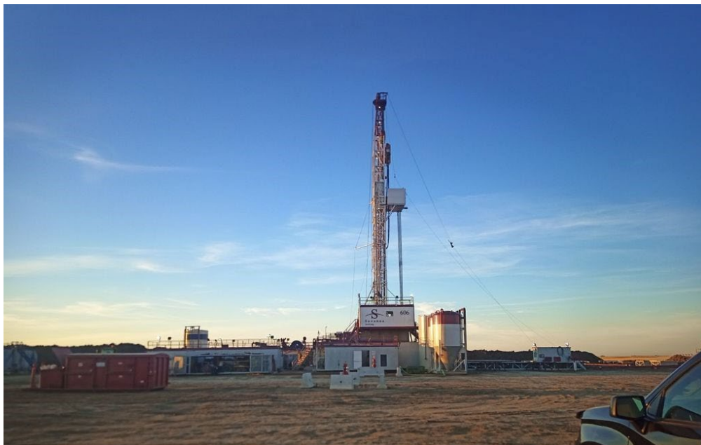
Figure 1: Drilling Well #3 on Pad #1. Well #1 and Well #2 can be seen in the foreground of the drilling rig
